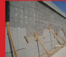
I-215 On-Ramp to Southbound I-15 Ramp widening Salt Lake County, Utah, USA
